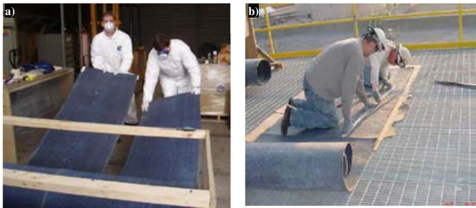
Fig. 4. Typical technology of insulation with aerogel: a) storage in rolls; b) installation and fixing with staples
